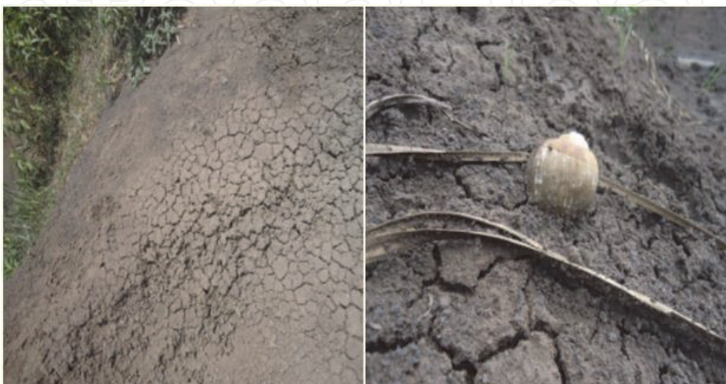
Figure 9. Highly expansive materials with numerous surface cracks. Photo credit, Nseka, march 2019.
