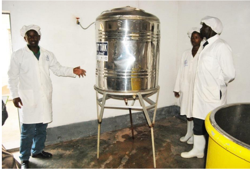
Figure 5. Water treatment system (450lt capacity)
